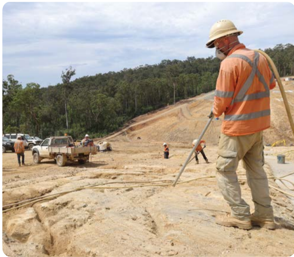
LABOURING LEGEND: Bodalla local and gun on the ground, Jason Bryan, cleans out a seam of the dam wall foundation with high-pressure air.
