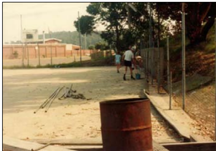
Narooma Rotary Club dismantles the fencing around the open-air skating rink ready for the construction of the Sport and Leisure Centre. (Photo courtesy Narooma Rotary Club).
