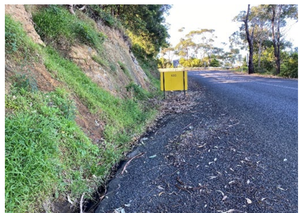
Photo 41: View east along Bermagui Road showing steep slope on northern side of road and exposed orange-brown clays
