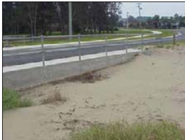
Figure 5-1 Sand covered outlets of culverts under McLeod Street
