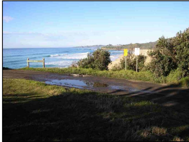
Figure 7: Poor drainage at Duesbury Car Park
