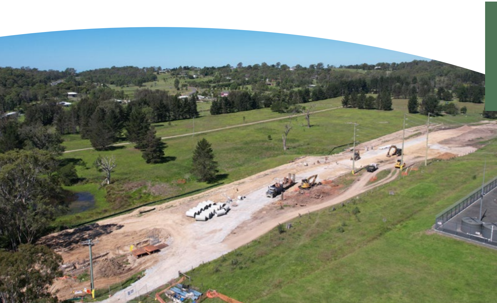
Image: Work has commenced on the access road to south Moruya that will support the development of new homes in the future. This project is a part of the Moruya Housing Infrastructure project.
