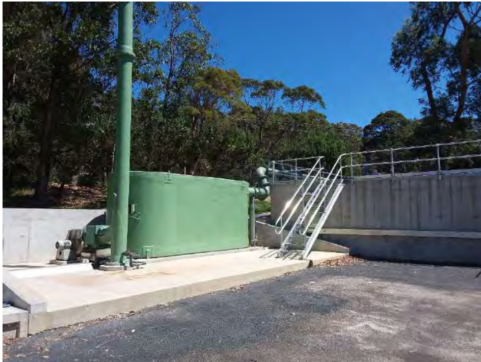
Figure 13 - 4: Tomakin STP Bioreactor
