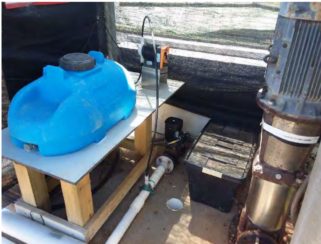
Figure 16 - 6: Narooma STP – Sodium Hypochlorite Container
