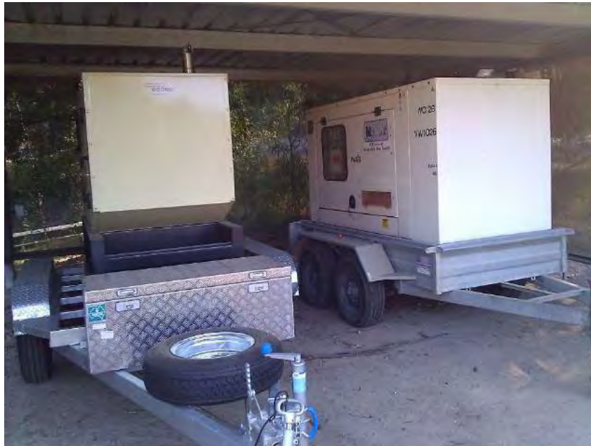
Figure 6 - 3: Diesel Generators Stored at Batemans Bay STP
