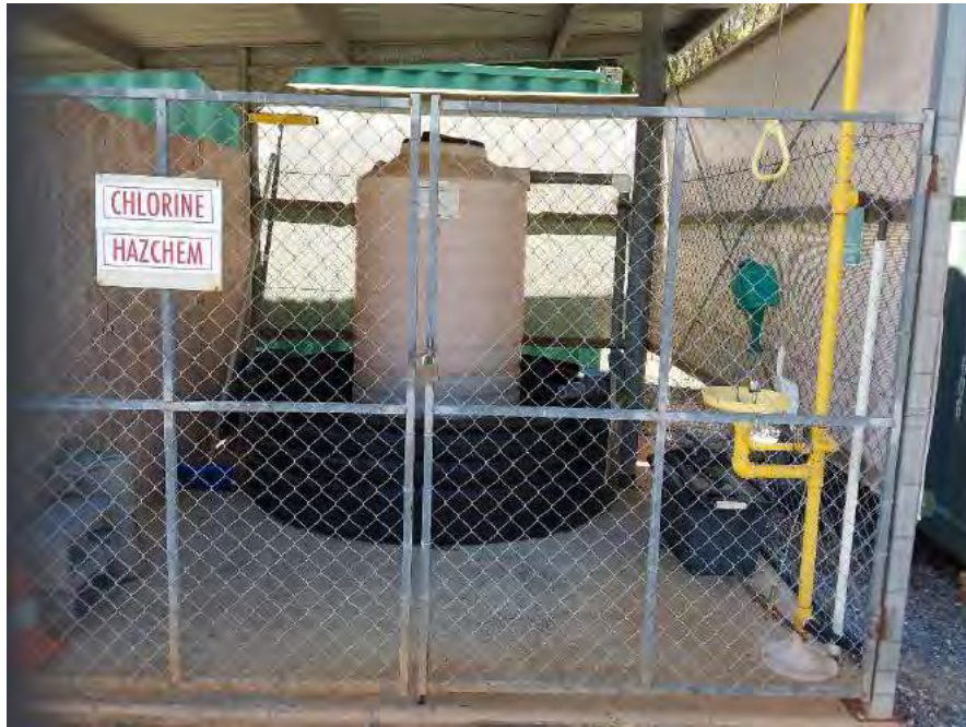
Figure 16 - 5: Narooma STP – Chemical Storage for Sodium Hypochlorite
