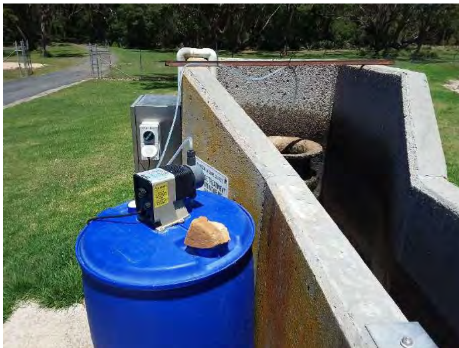
Figure 15 - 4: Tuross STP – Chemical Storage for Alum Sulphate
