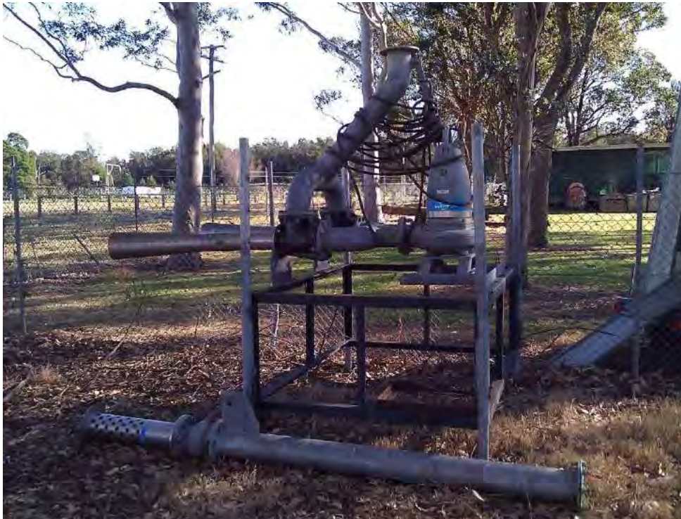
Figure 12 - 2: Ejectors Used in Batemans Bay STP
