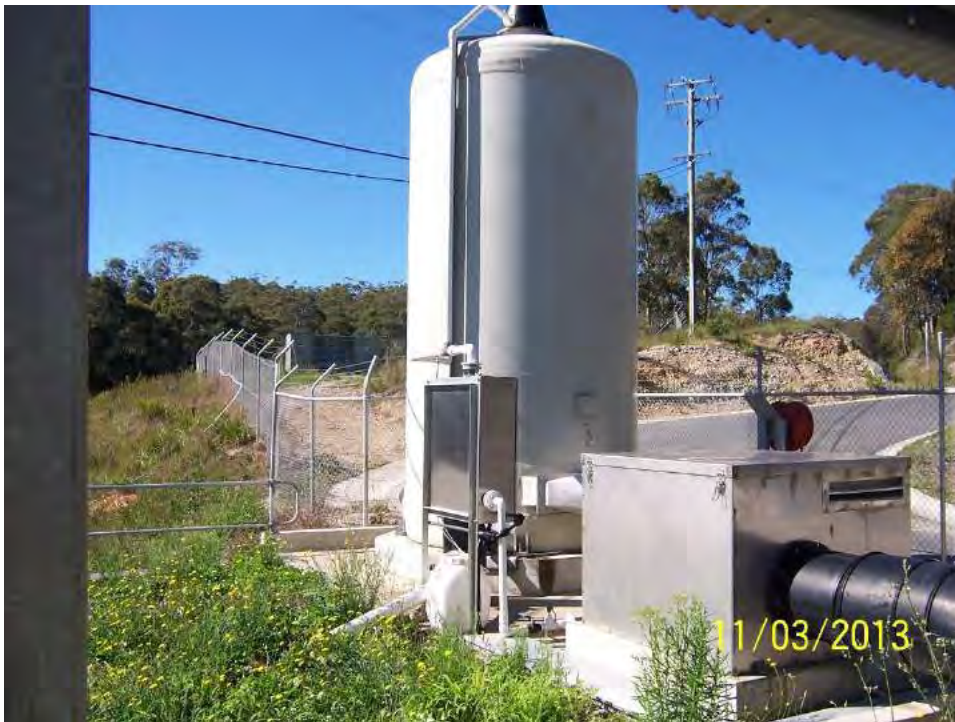
Figure 12 - 6: Odour Treatment Bioreactor System in the Batemans Bay STP
