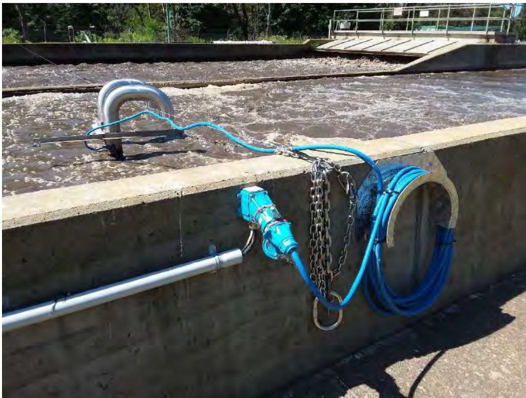
Figure 16 - 3: Ejectors Used in Narooma STP
