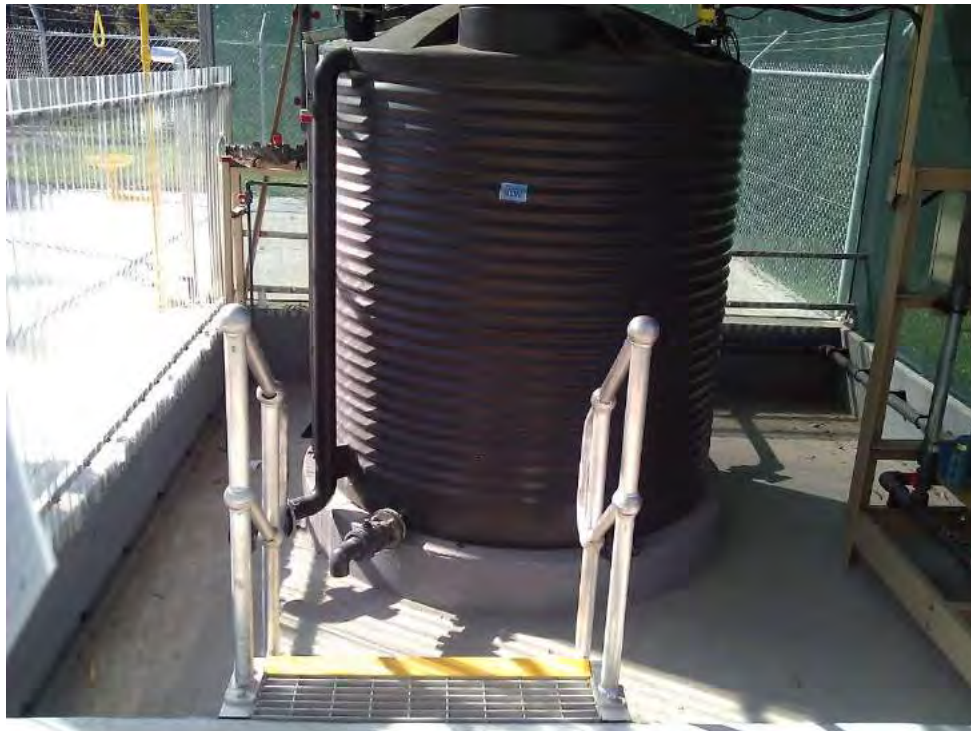
Figure 12 - 5: Batemans Bay STP – Chemical Storage Sodium Hypochlorite
