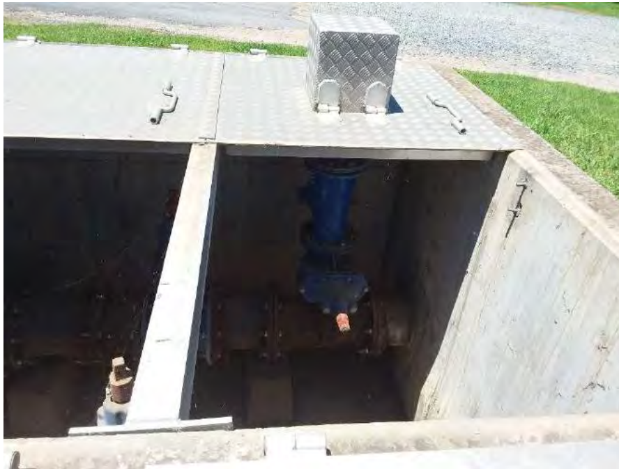
Figure 6 - 6: Typical Installation for Sykes Pump Bypass
