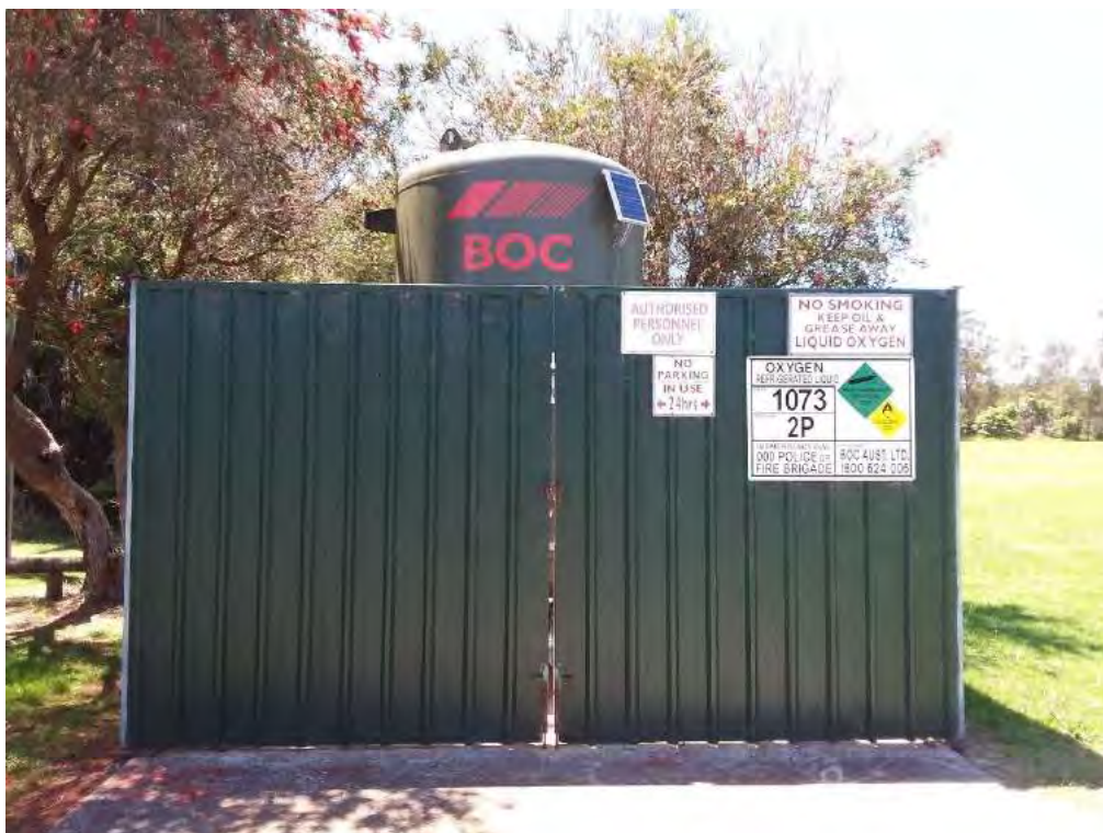
Figure 12 - 7: Pure Oxygen Used for Odour Treatment in the Batemans Bay Sewerage Scheme
