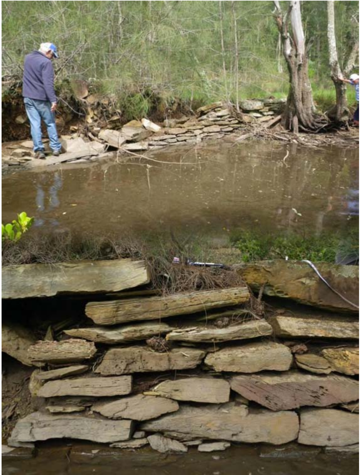
Upper picture: Arthur Andy next to the section of collapsed wall. Lower picture: detail of stone wall construction.
