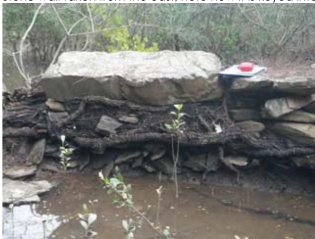
Detail of stone wall from southern side, showing presence of large tree roots.
