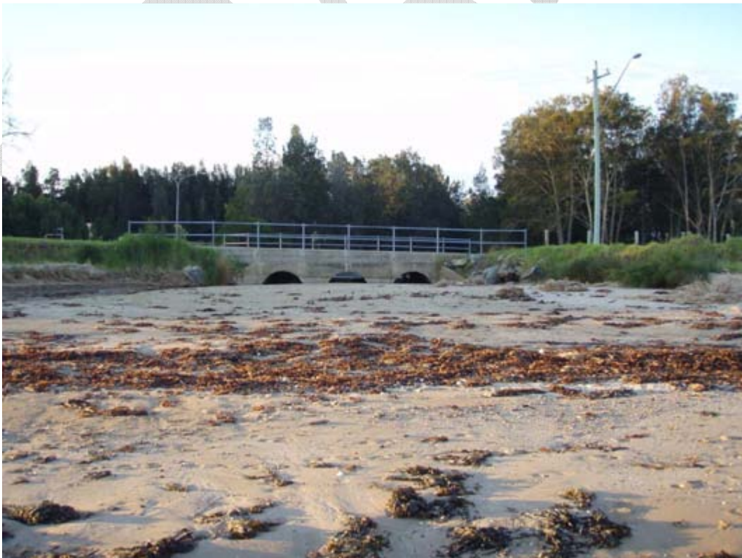
Figure 3.18 – Visible erosion along McLeod Road damaging bridge's seawall protection and pipes under bridge covered with sand (March 15 th 2010)
