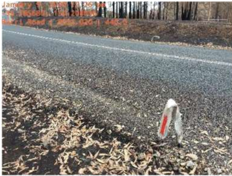
Fire damaged guide posts on both sides of Burri road (Malua bay)
