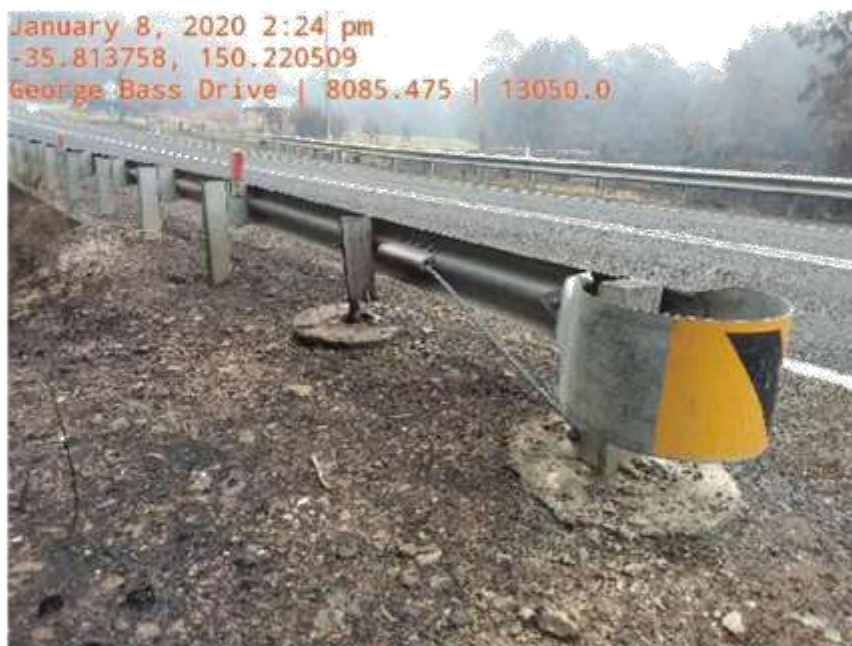
Fire Damaged guard rail along George Bass Drive
