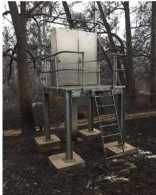
Fire impacted on the 5 bores and associated electrical equipment. Extent of damage is still being assessed.
