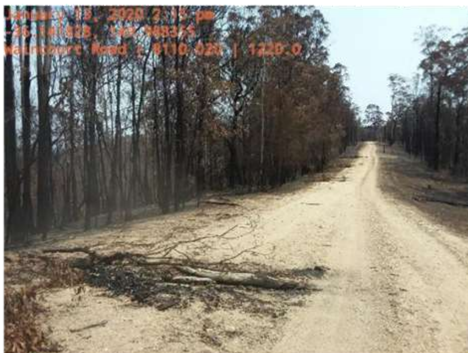
Waincourt Road, fire effected tree line neighbouring roadside making the road unsafe
