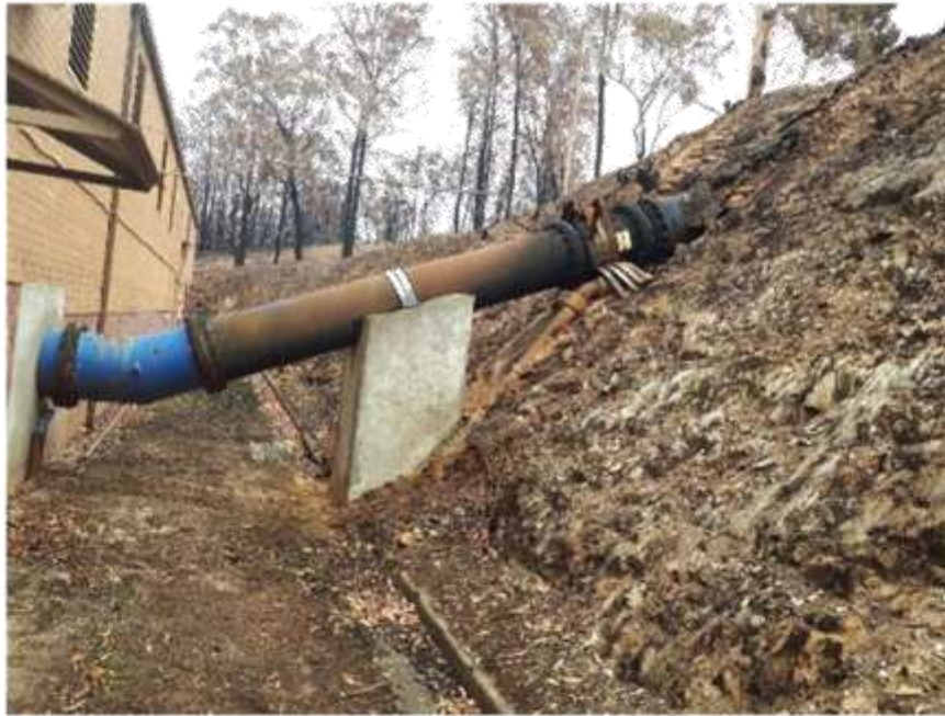
600mm flow meter on the pumping line to the NWTP has been impacted by fire and requires replacement.
