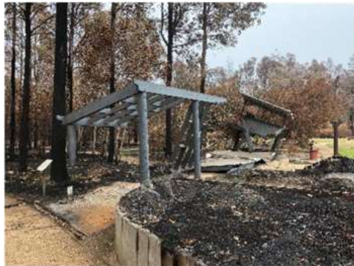
Damage to wooden structures such as bird shelters, green houses and playground equipment
