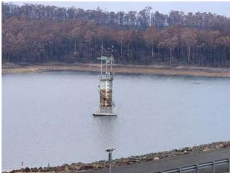
Roof to the tower has come away from the structure, suspected to have been blown off. Damage to the aeration system is currently
