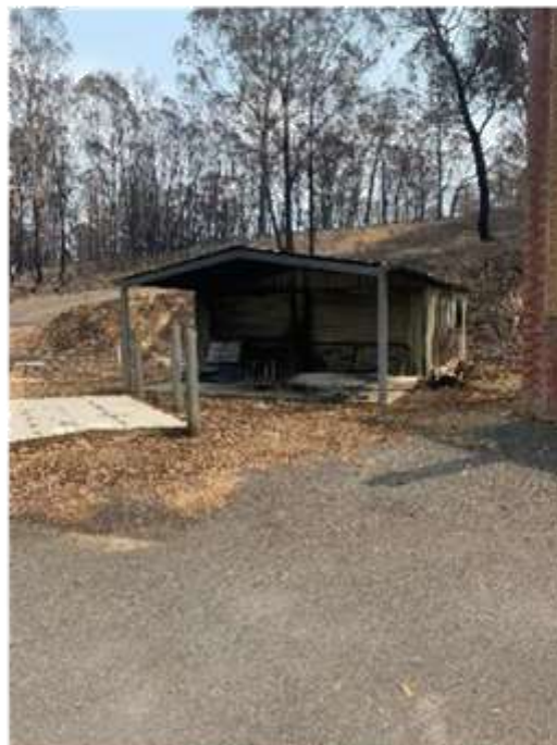
Colourbond shed at Deep Creek Dam has been destroyed. No Council assets are believed to have been stored in the shed at the time of the fires.
