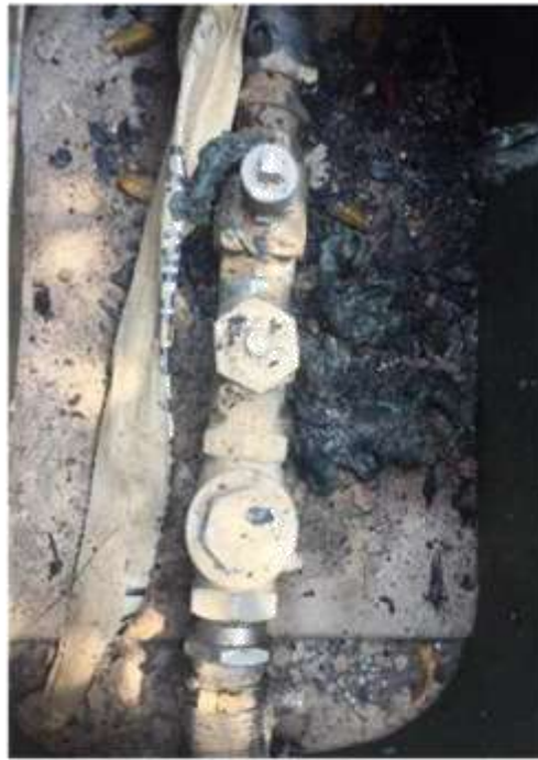
Example of damaged boundary kit
