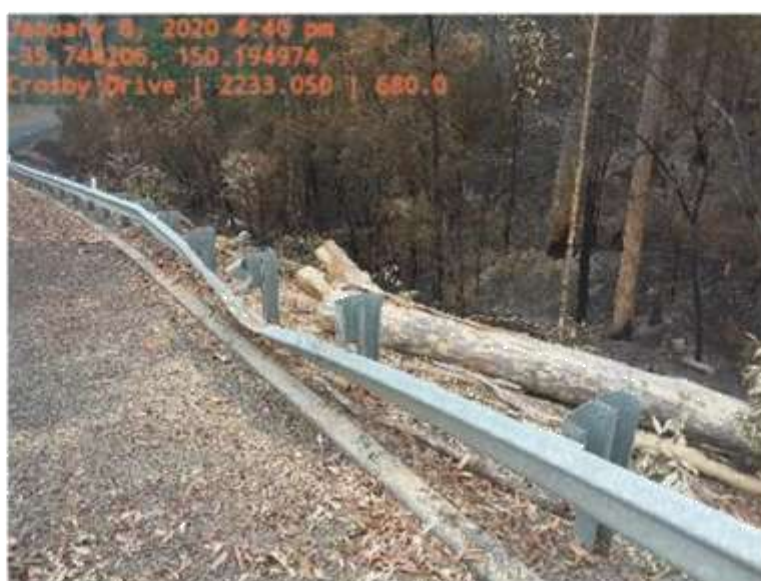
Crosby Drive, fire damaged tree fell on guardrail
