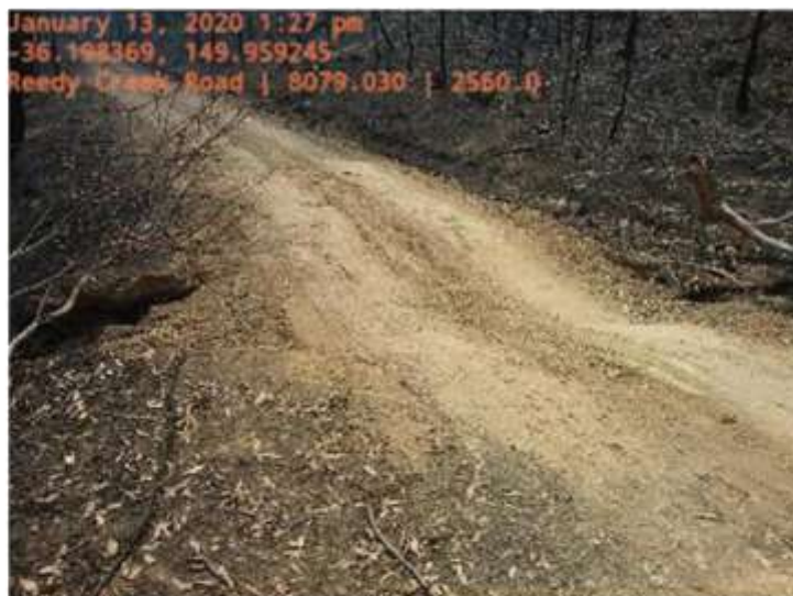
Complete pipe collapse due to fire damage along Reedy Creek Road
