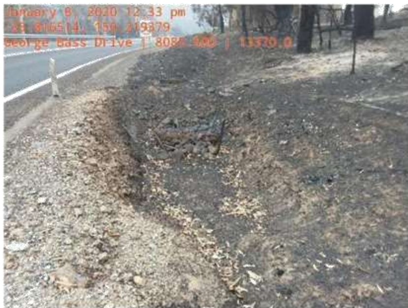
George Bass Drive, culvert fire damage
