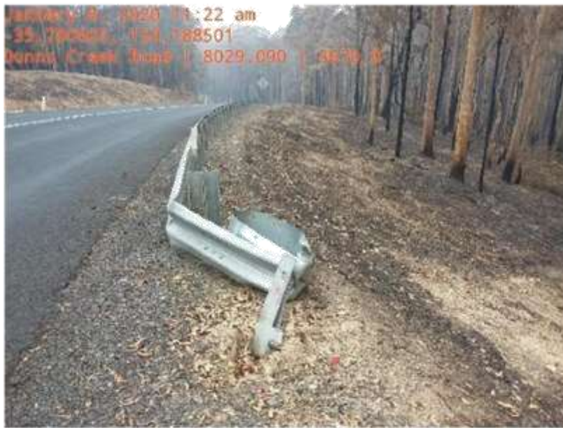
Guardrail damaged from falling tree along Dunns Creek Road
