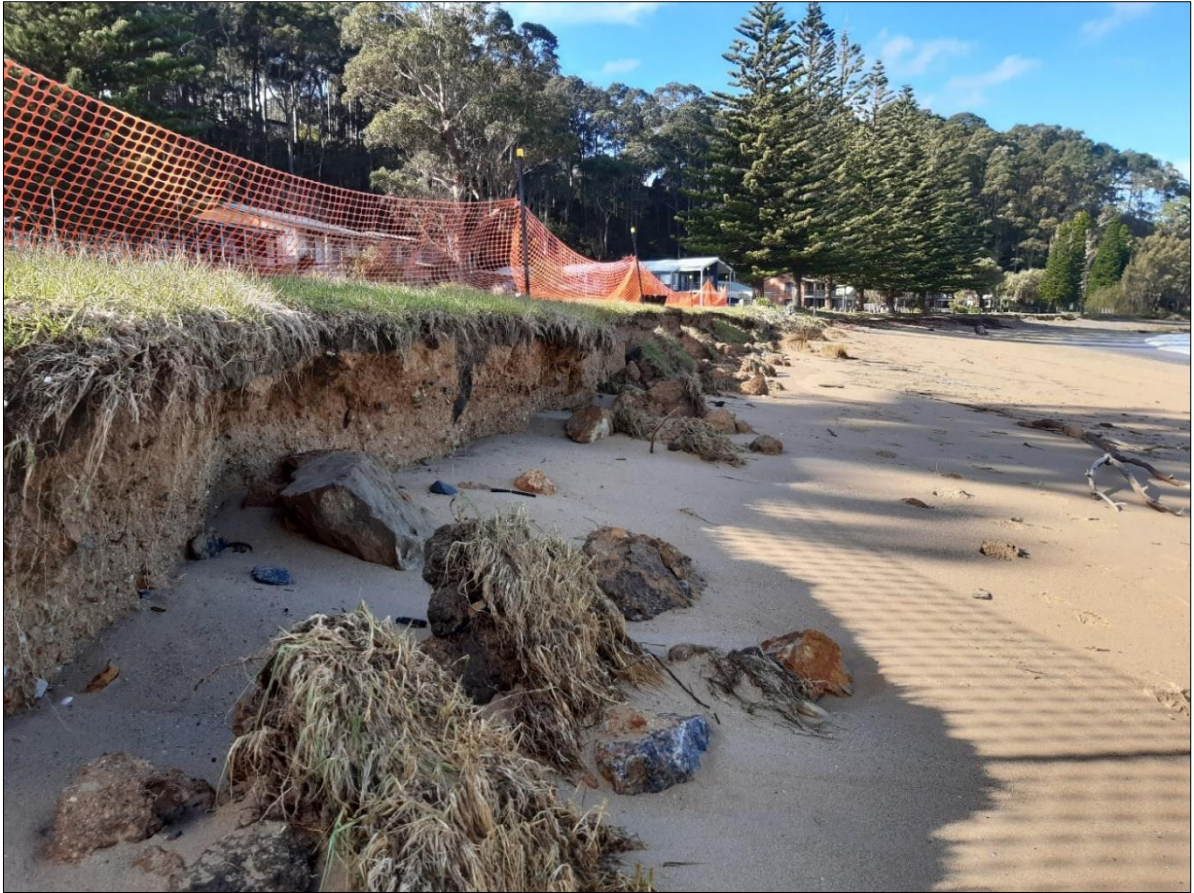
Image 6: Erosional impacts on the dune and adjacent Bay Road.
