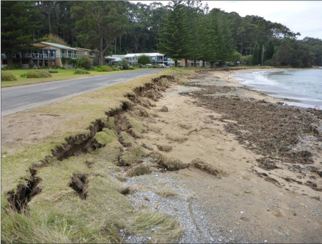
Image 4: Photo looking east illustrating the undermining of the existing bank from coastal processes.
