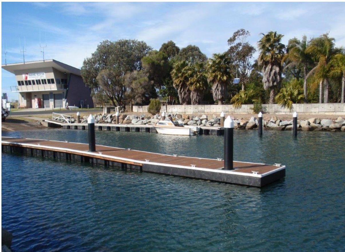
New pontoons at the highly used regional boat ramp at Hanging Rock, Batemans Bay
