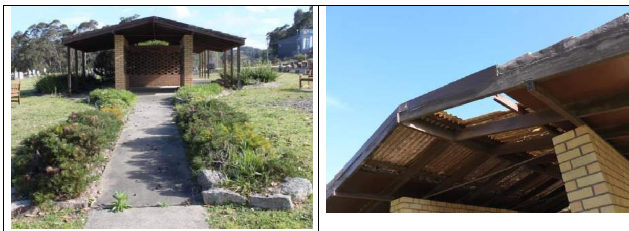
The Batemans Bay columbarium needs maintenance
