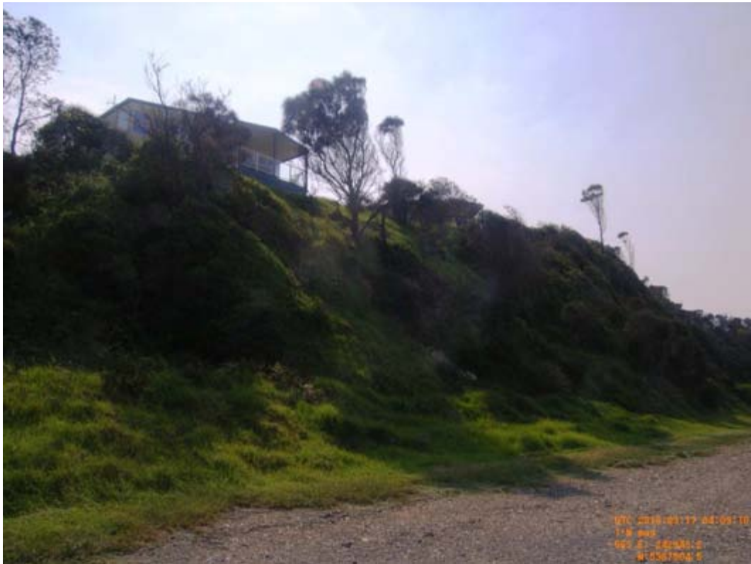
Figure 3.71 – Cabins close to the edge of the cliff near Narooma SLSC (March 17 th 2010)
