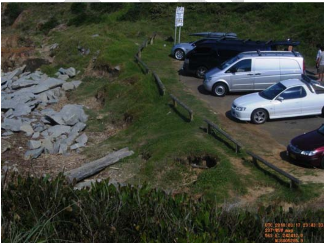
Figure 3.60 – Erosion in front of carpark at One Tree Beach south (March 18 th 2010)
