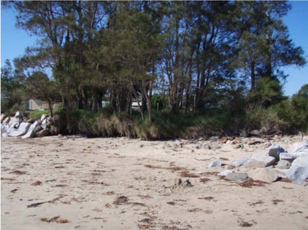
Figure 3.33 – Undercutting of trees where no protection at Casey Beach (March 16 th 2010)
