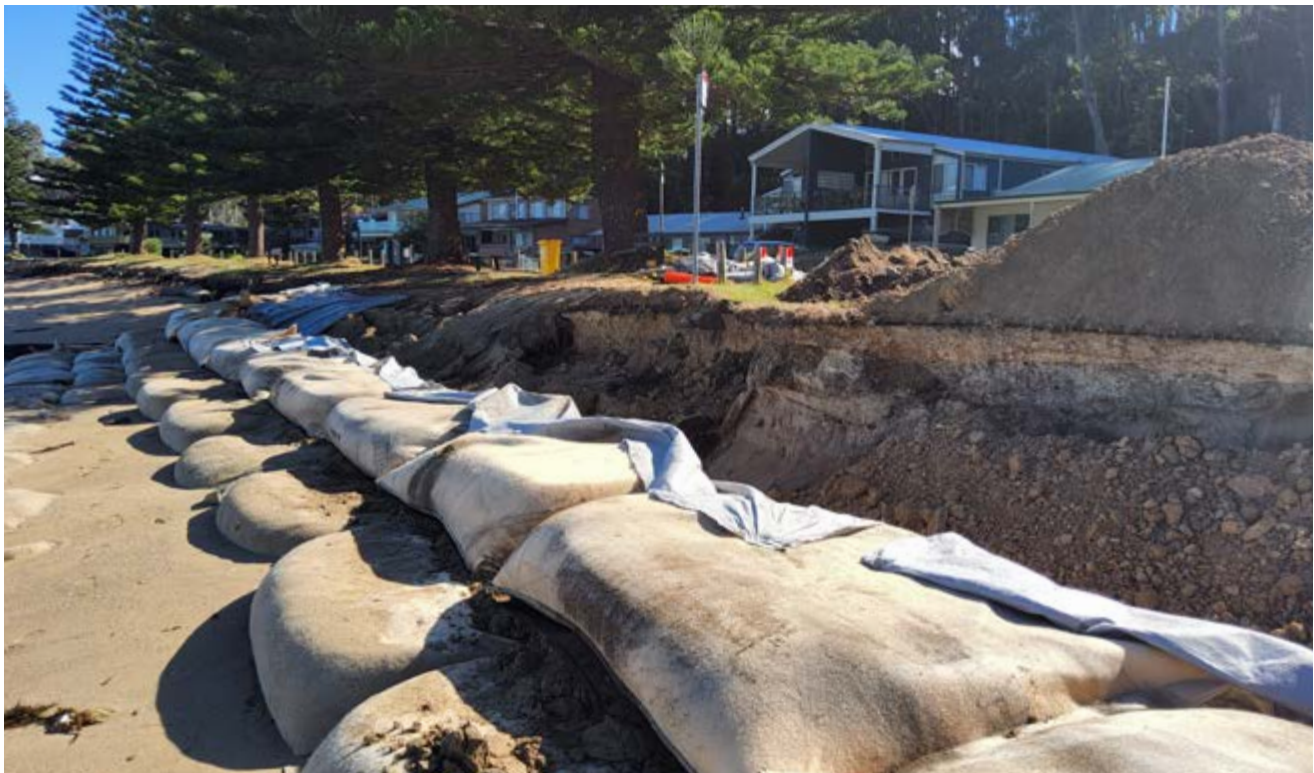
Image: A sandbag structure protects the shoreline at Long Beach, part of the Eurobodalla Open Coastal Management Program
